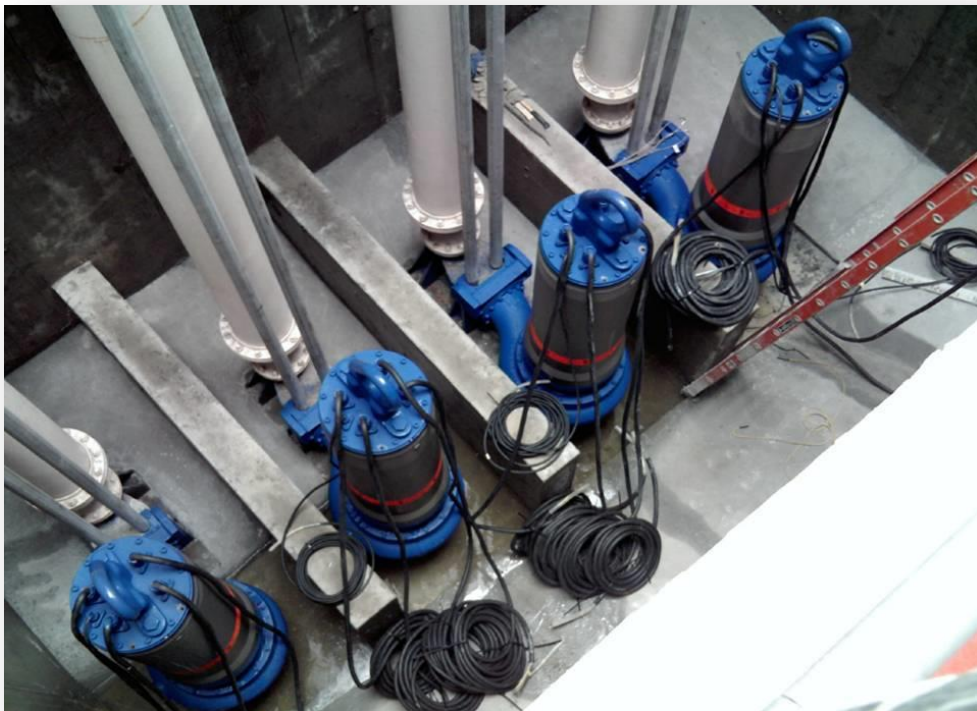
Wet-pit Submersible Pumps –North Fork Sewage Pumping Station-
