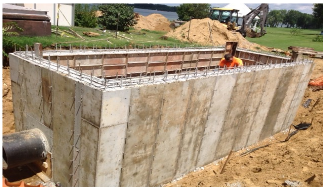
Pictured above is the Janalee Drive SPS Flow Meter Pit Henderson, Kentucky
