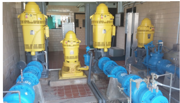
Pictured above is New High Service Pumps Water Treatment Plant Livingston, Tennessee
