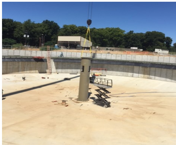
Pictured above captures setting the column of the 160 ft. diameter Final Clarifier North Wastewater Treatment Plant Henderson, Kentucky
