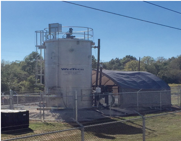
Pictured above is Solids Contact Clarifier and Membrane Filtration Pilot Testing South Water Treatment Plant Henderson, Kentucky
