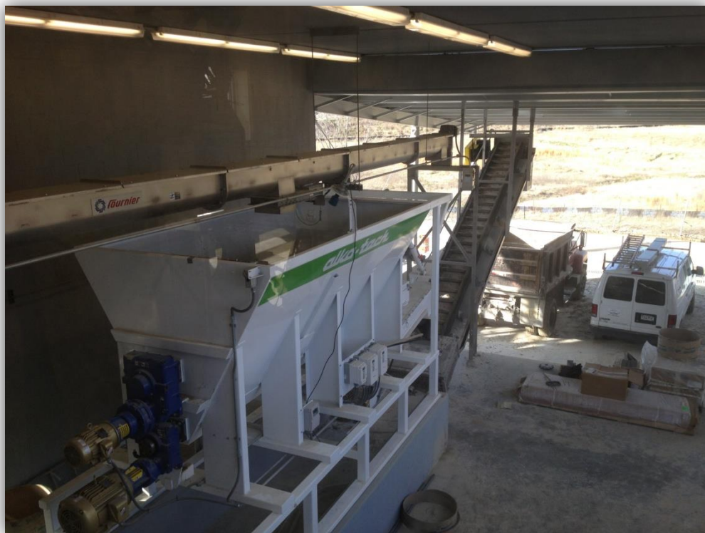
Cement Kiln Dust Cake Sludge Processor Lewisburg Wastewater Treatment Plant Lewisburg, Tennessee
